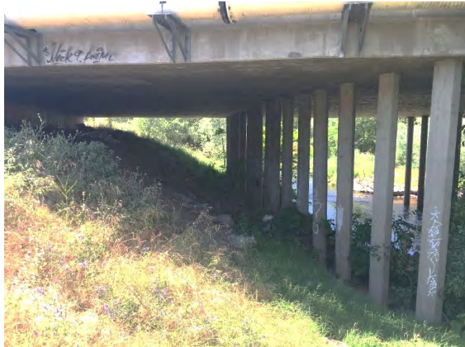
Photo 4-5: End slope at south abutment of Atkinson Street Bridge over Dry Creek.
