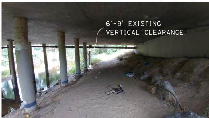
Photo 4-9: Existing graded area at the south abutment of the Vernon Street Bridge, looking west.
