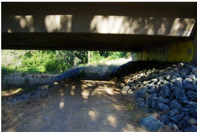
Photo 4-3: Existing graded area under Cook Riolo Road Bridge at north abutment, looking west.
